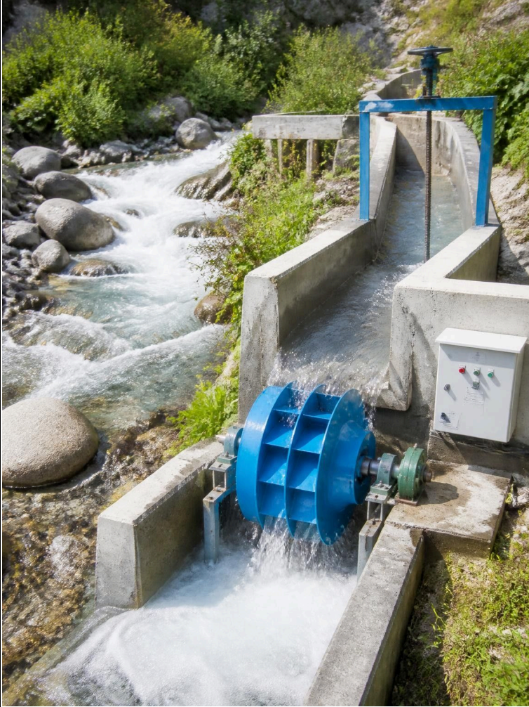
Low-impact stream hydel plant.
